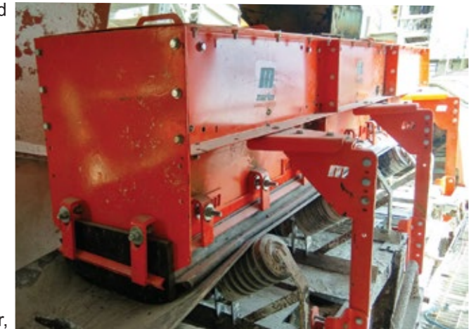
ECO settling zone
